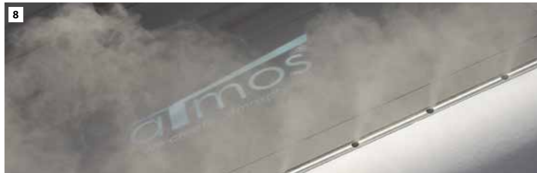
++ Hygienic, biological air ventilation system inside the facility
